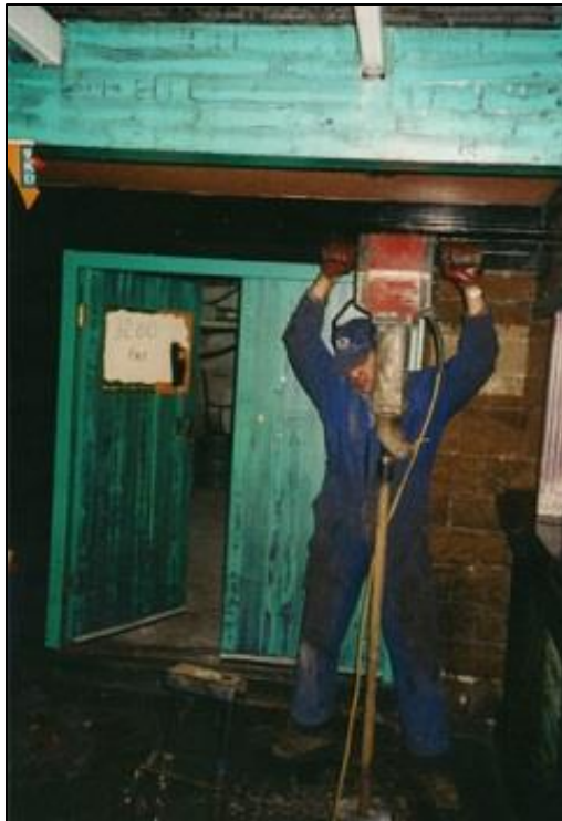
Follow on soil sampling through diamond core hole with 110 volt electric percussion hammer to avoid fumes and gain access to difficult drilling locations
