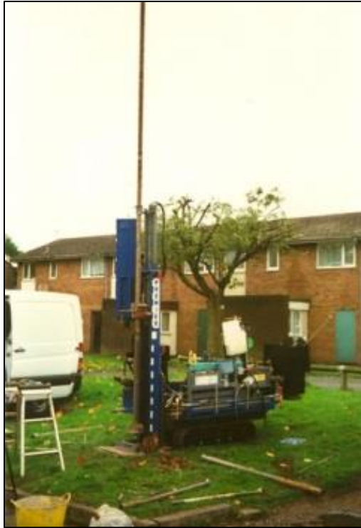
Rubber Crawler Tracked One Ton Petrol Powered SPT Drop-Hammer Swing away drill carriage with 8.0 metres of rods jacked in the air (to speed drill tool change over)
